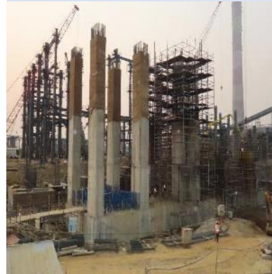
Unit #3 - Turbine Generator Deck
