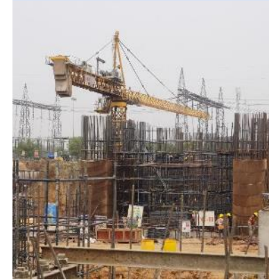
Unit #3 - Turbine Generator Deck
