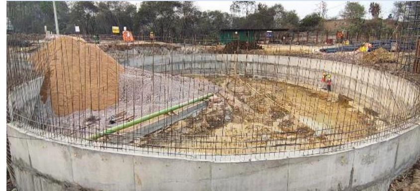
High-Rate Solid Contact Clarifier
