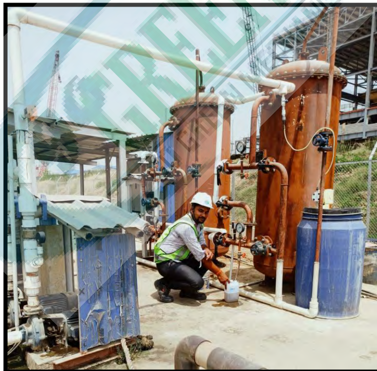
Figure 12: Water Sampling at STP Outlet township
