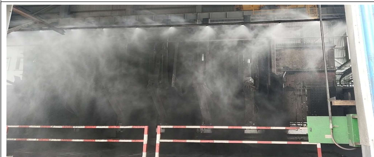
SPRINKLER SYSTEM AT WAGON TIPLER
