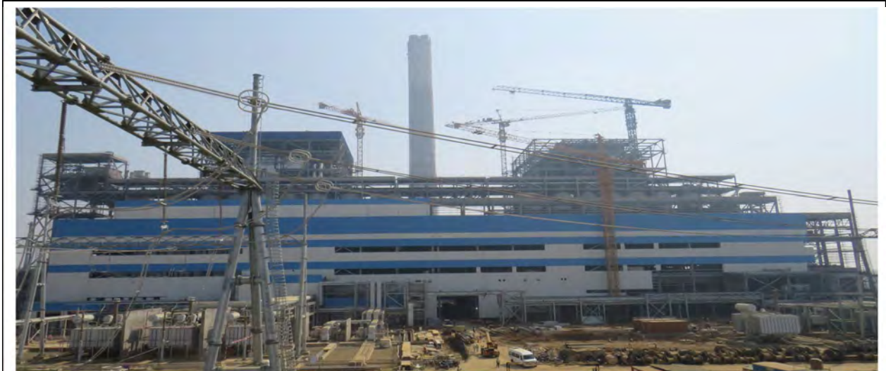
Main Plant View
