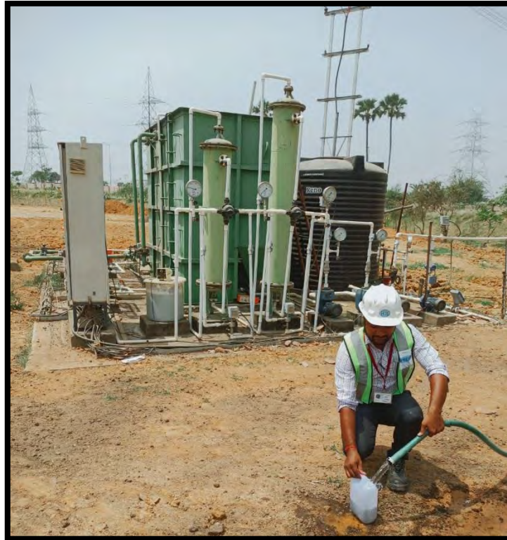
Figure 11: Water Sampling at STP Outlet plant
