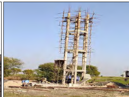
Water Tank - Barla
