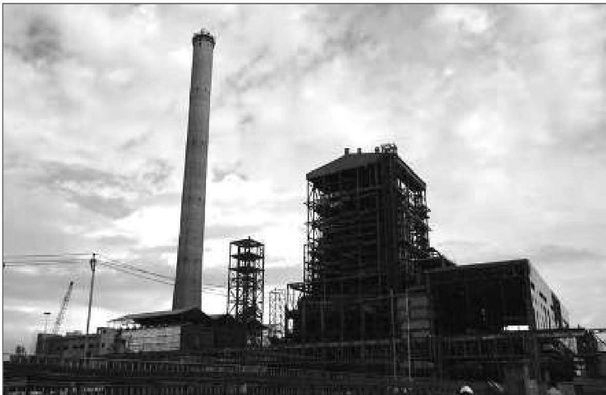
Figure No.1. Korba West Power Company Limited (KWPCCL)
