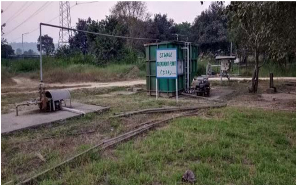
Sewage Treatment Plant at Mahan Energen Limited
