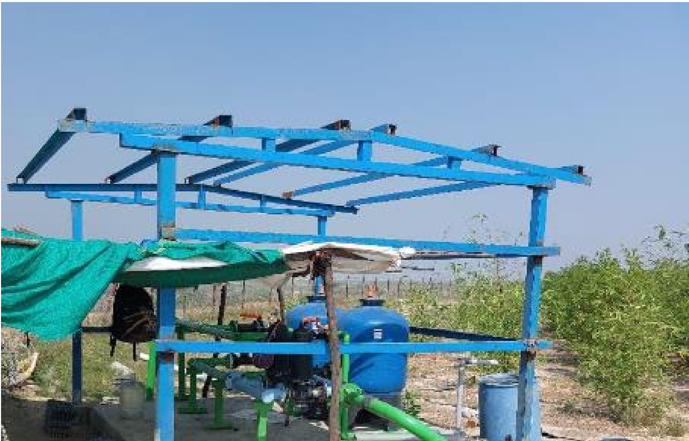
Drip Irrigation system-buster pump, Filtration units
