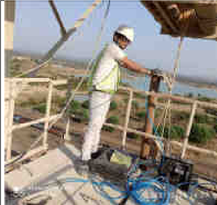
Fly Ash Silo No.2 (Inlet)
