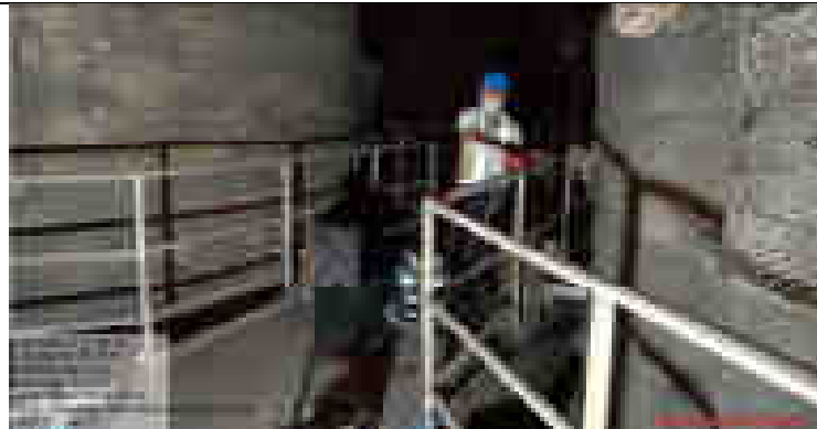
Unit#1 Boiler Duct Pass- A
