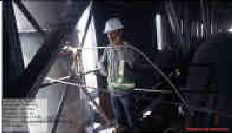
CHP Crusher Duct Extraction Pass -A
