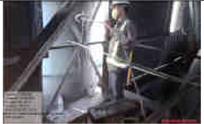
CHP Crusher Duct Extraction Pass -B
