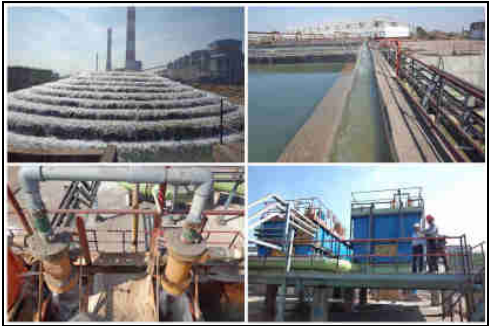
FIGURE 5.15 (b) : VIEW OF WATER TREATMENT PLANT AT TIRODA TPP (5x660 MW)
