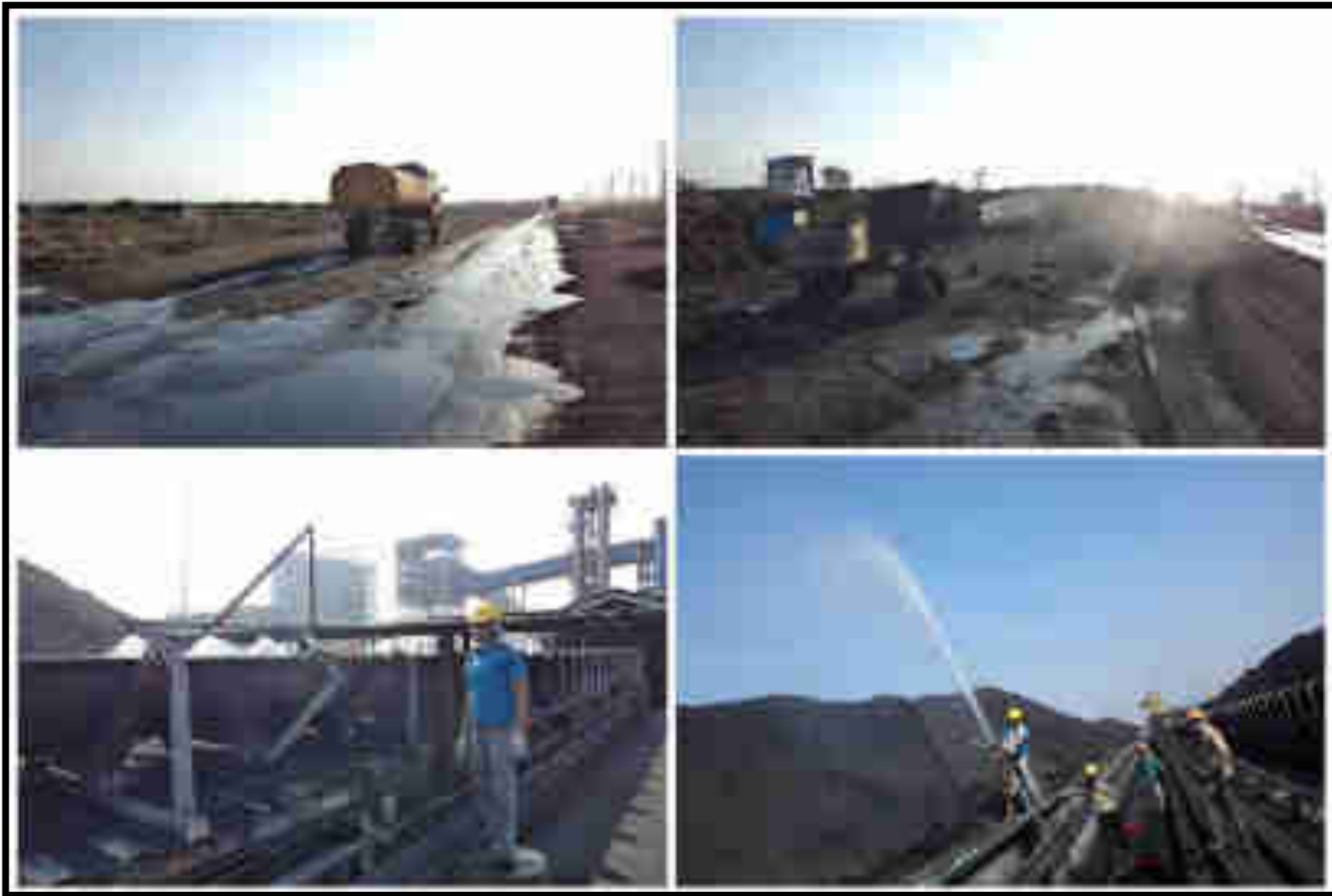
FIGURE 6.0(b) : CTBD & OTHER WASTEWATER BEING USED IN COAL HANDLING PLANT AT TIRODA TPP (5x660 MW)
