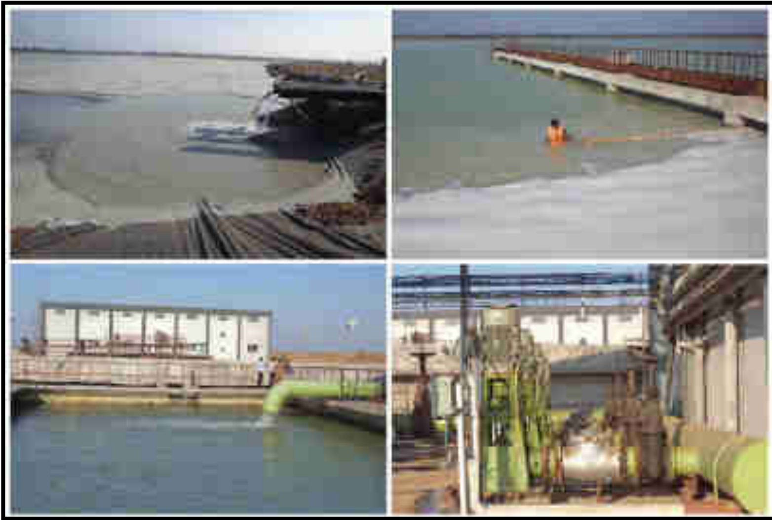
FIGURE 7.1 : VIEW OF ASH WATER RECOVERY SYSTEM AT TIRODA TPP (5x660 MW)
