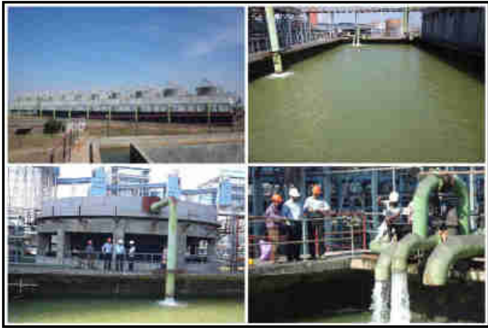
FIGURE 6.0(a) : CTBD BEING USED IN ASH HANDLING PLANT AT TIRODA TPP (5x660 MW)
