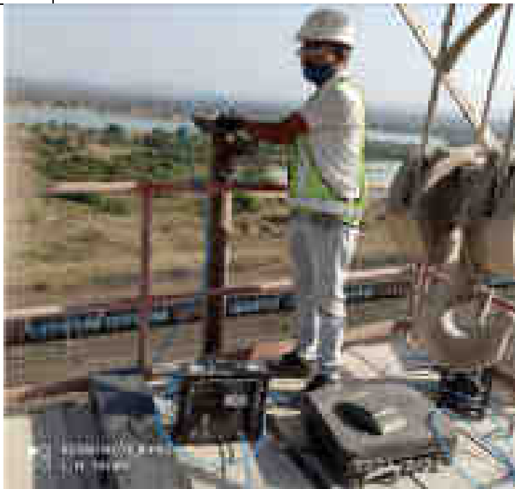
Fly Ash Silo No.1 (Inlet)
