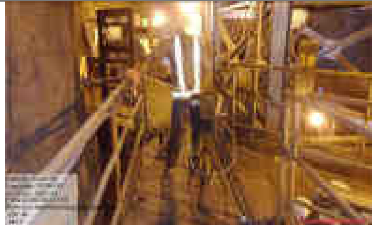
Unit#4 Boiler Duct Pass- A
