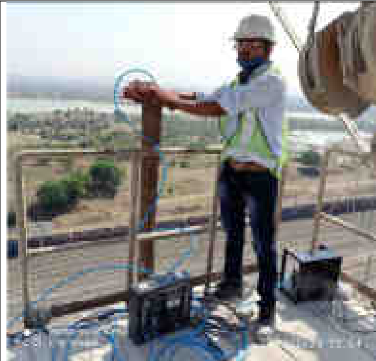
Fly Ash Silo No.5 (Inlet)
