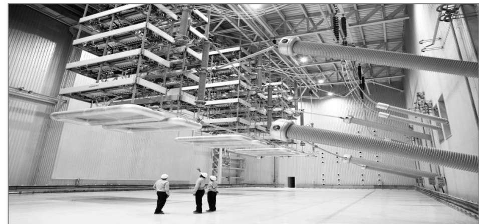
View of HVDC Transmission System
