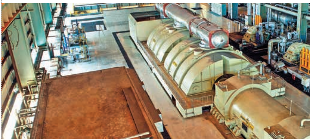
TG Floor of one of the operating units.
